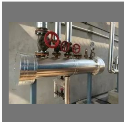
Duct Insulation Service
