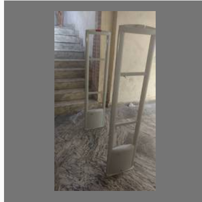
Security Alarm System
