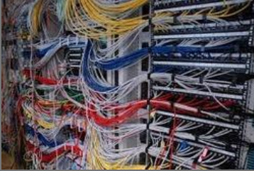
Servers & Network Configuration
