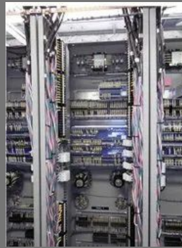
SCADA Installation Services
