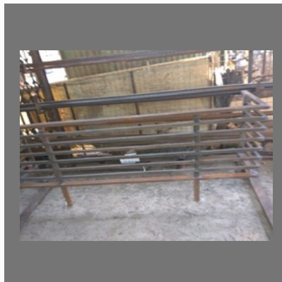
Steel Iron Railing
