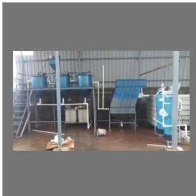
Sewage Treatment Plant Service
