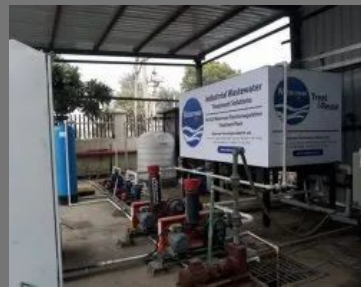
Industrial Wastewater Treatment Plant
