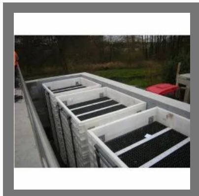
Decentralized Sewage Treatment Plant
