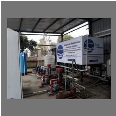
Effluent Treatment & Wastewater Treatment Plant
