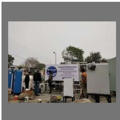
Wastewater Treatment Plants Service
