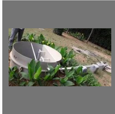
Domestic Sewage Treatment Plant
