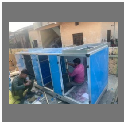
Wet Scrubbers Units
