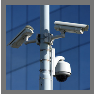
Industrial CCTV Systems
