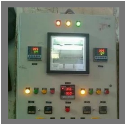
Air Control Panel
