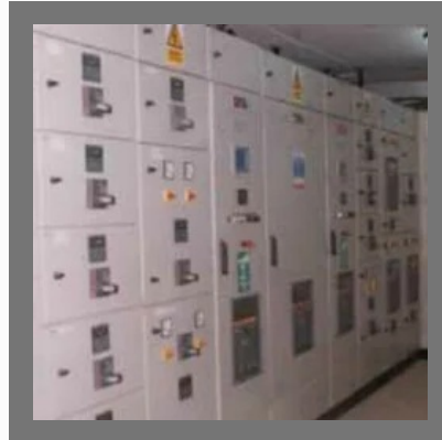
Main LT Control Panel
