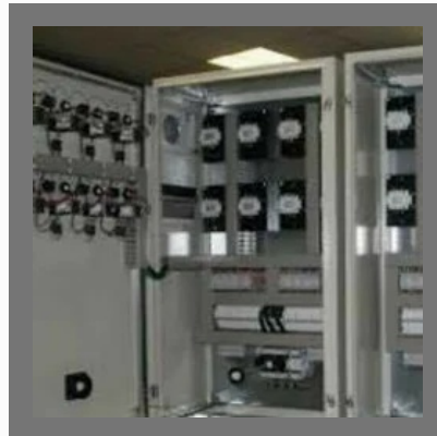
MVC Control Panel
