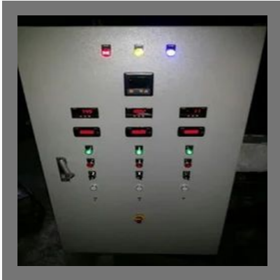
Electric Control Panel
