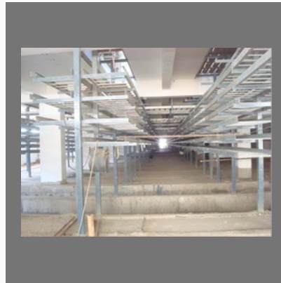
Industrial E&I Projects Material Procurement And Storage
