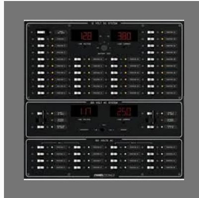
Electrical Paneling, Distribution IT Solution
