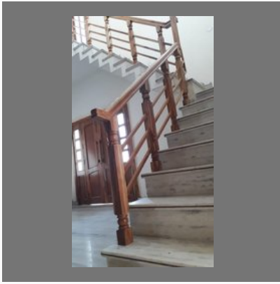
Wooden Hand Railing
