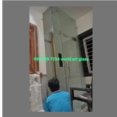
Bathroom Shower Glass Partition
