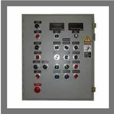
MCC Control Panels
