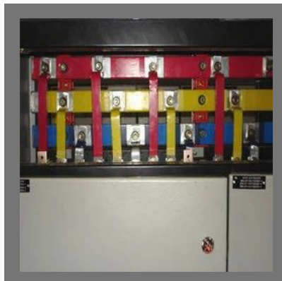
LT Control Panels
