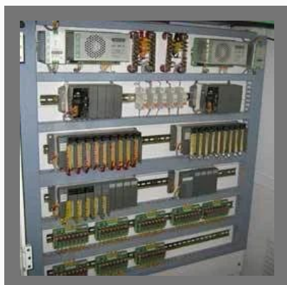
HT Control Panels
