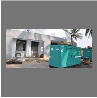
24x7 Full Power Backup
