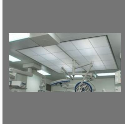
Ceiling Laminar Airflow
