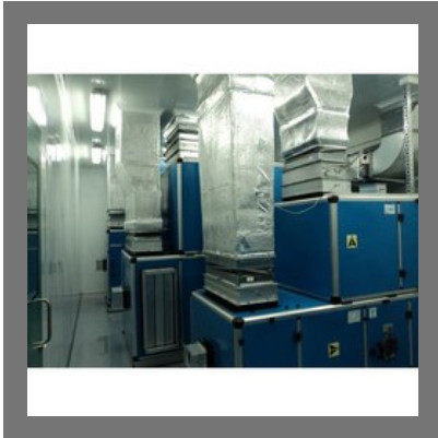
AHU With AC Ducting
