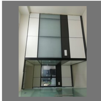
Steel Glass Door
